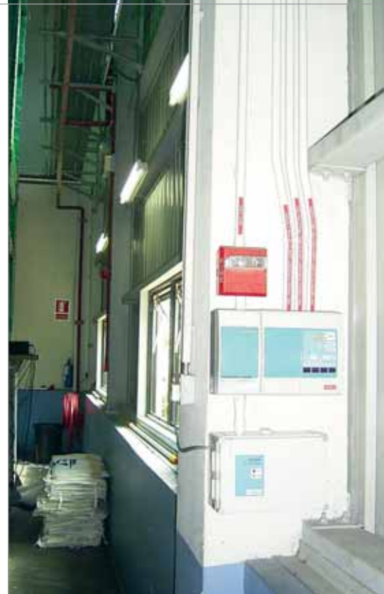
The Xtralis VESDA detectors are installed at shoulder-height for easy access for maintenance
